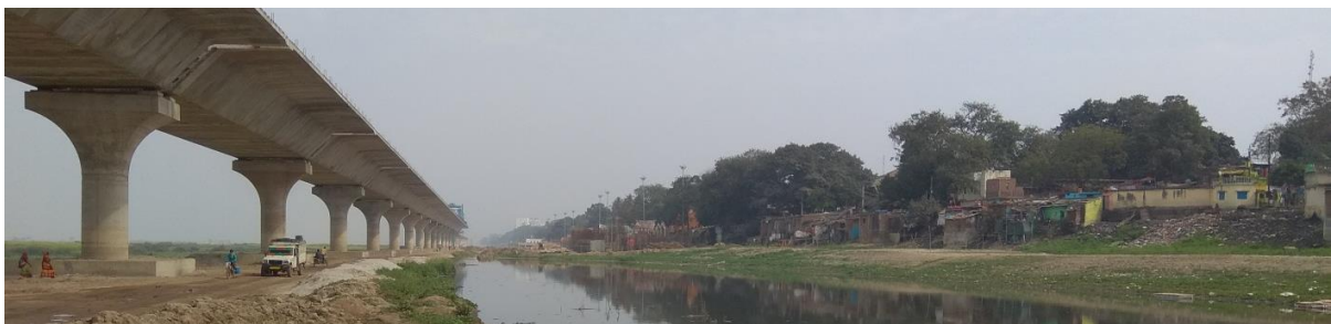
Figure 8: Construction of expressway causing narrowing of channel and wetland
